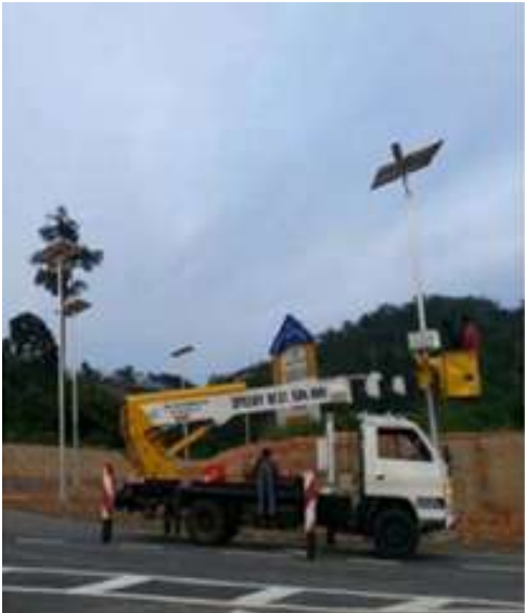
60w Solar LED Peng. Hulu, Perak, JKR KL
