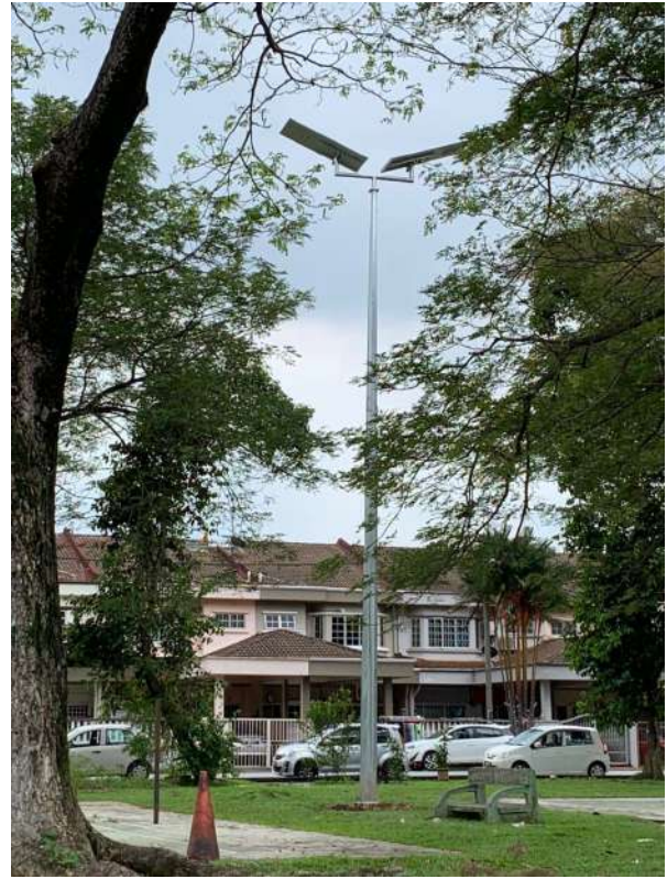
All in One Majlis Perbandaran Klang
