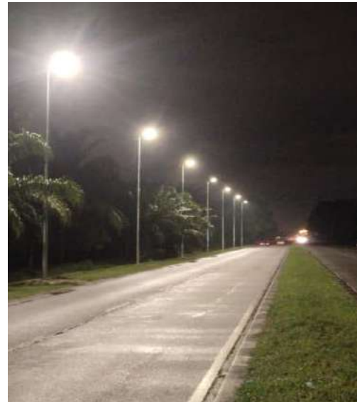
120w Solar LED Jalan Kapar, Klang, JKR Selangor
