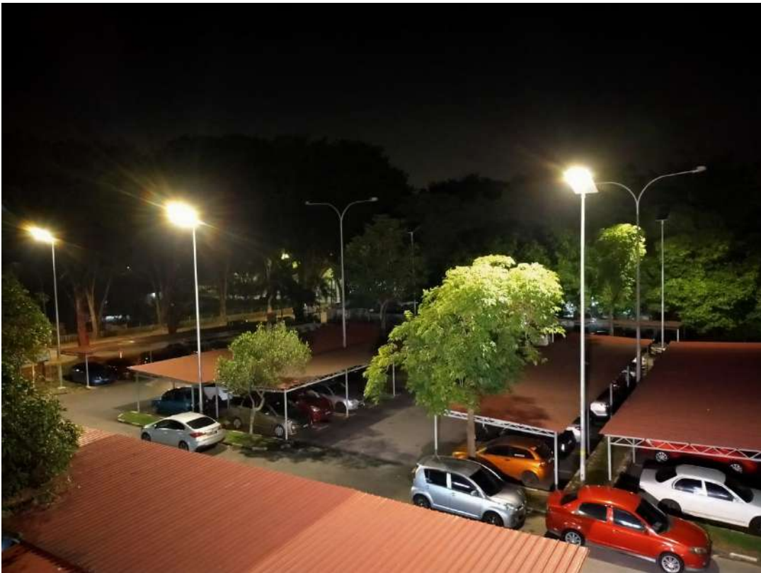
All in One Jkr Selangor Quarters
