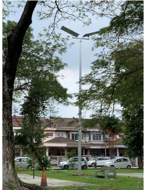
All in One Majlis Perbandaran Klang
