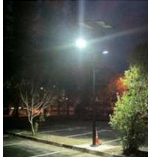
60w Solar LED Petronas Plant, Terengganu
