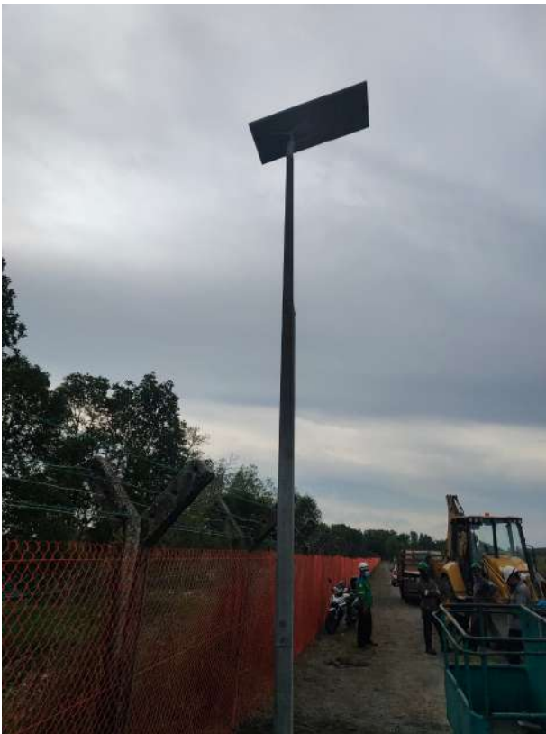
All in One TNB Station Kapar, Selangor
